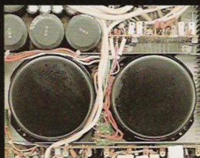
Separate right and left Toroidal power transformers used in SX-9100H/HB
